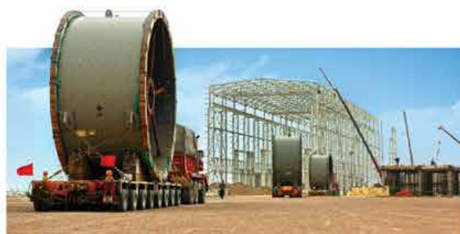
SANGAN 2.6 MTPA IRON ORE CONCENTRATE PLANT
